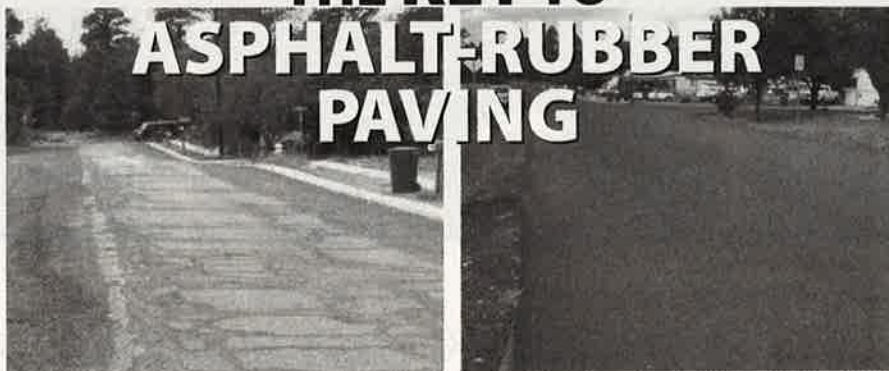
A Road in Flagstaff, Arizona before paving with Rubber/asphalt concrete modified with VESTENAMER® trans-Polyoctenamer.
